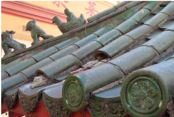
Figure 4.41 Some broken tiles on the eastern bay.
