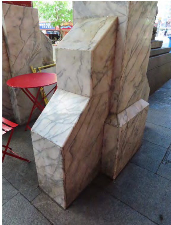
Figure 4.27 Chipped marble plinth.
