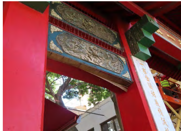
Figure 4.33 Peeling plyboard beneath decorative panel D.
