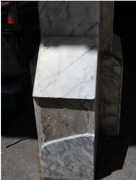
Figure 4.26 Broken marble plinth.
