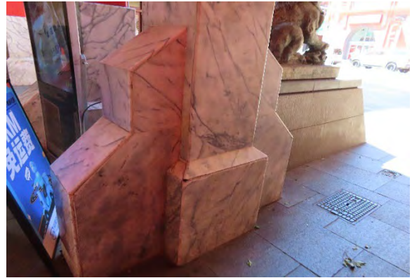
Figure 4.52 Chipped marble plinth.
