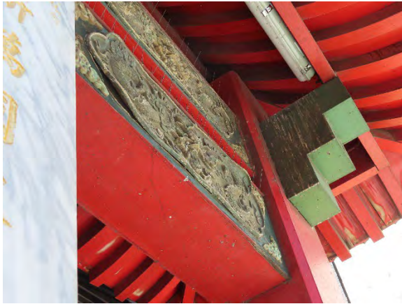
Figure 4.8 Fibreglass decorative moulding fixed to the panel E at the western bay of the secondary gate is distorted.
